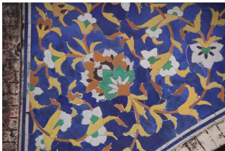
Figure. 11. Spandrels of the side arches decorated with arabesque designs in the technique of faience mosaic with Islamic color scheme (Source: Photograph taken by the author on 20 th December, 2018)
